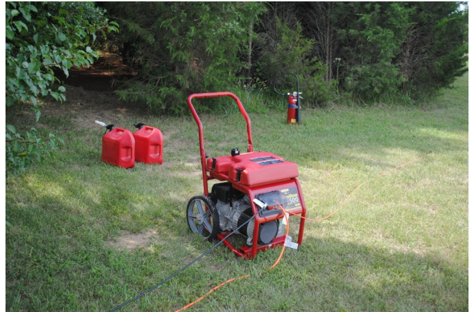
Figure 2: Big Gen for Station 2 and VHF
